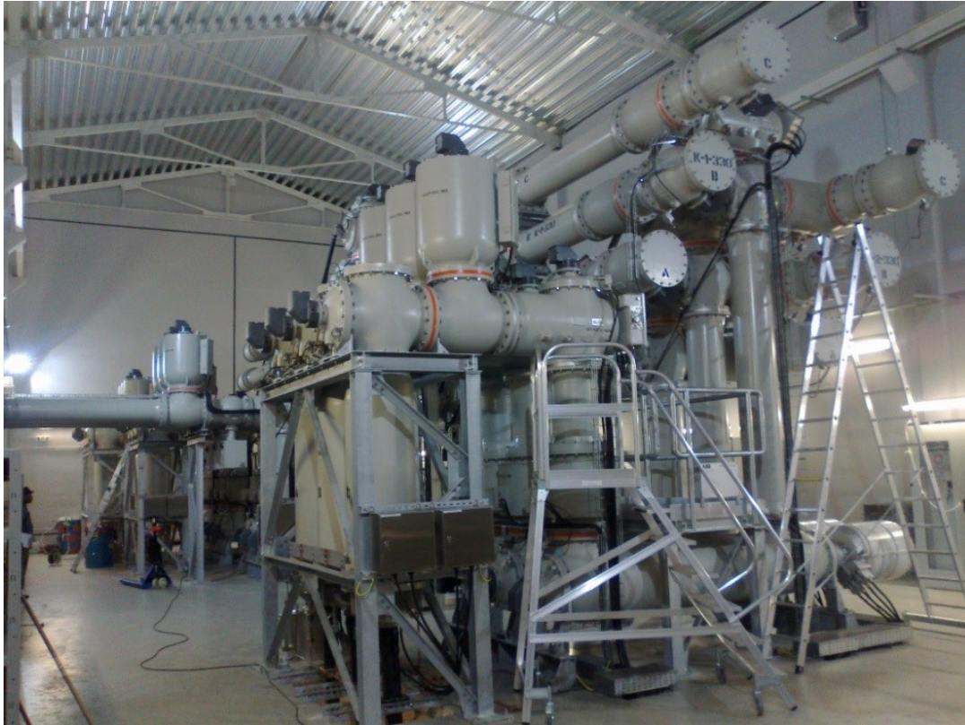
330kV substation "RigaCHP1" Gas-insulated switchyard
