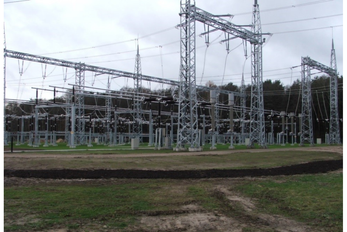
330kV substation "Imanta" Outdoor switchyard
