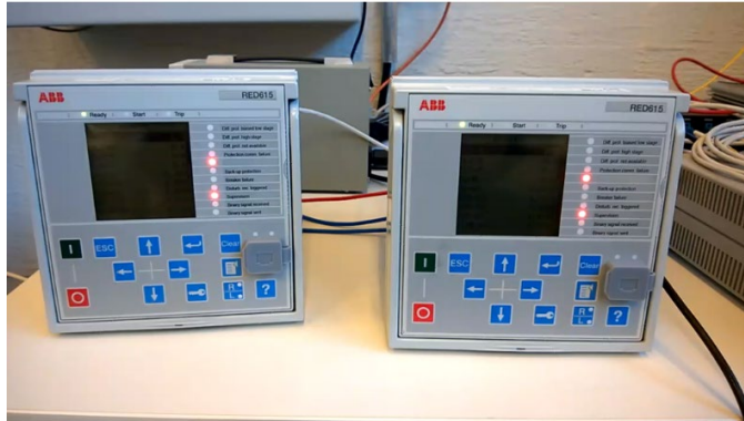
Relays connected to the test network
