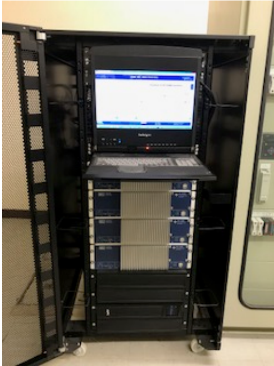
Centralised ANM System
